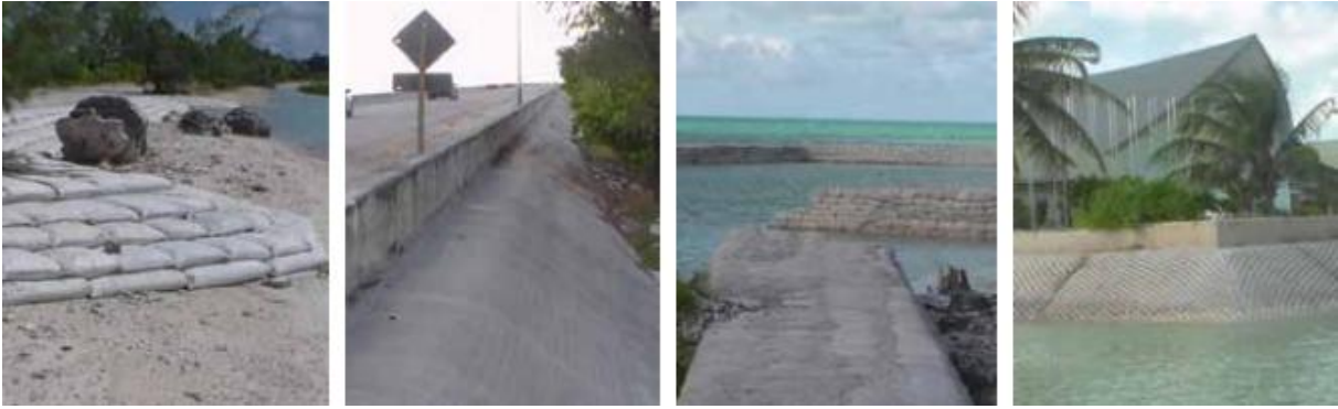
Figure 2: Sea wall structures in Kiribati ( Source: Paeniu et al., 2015)
