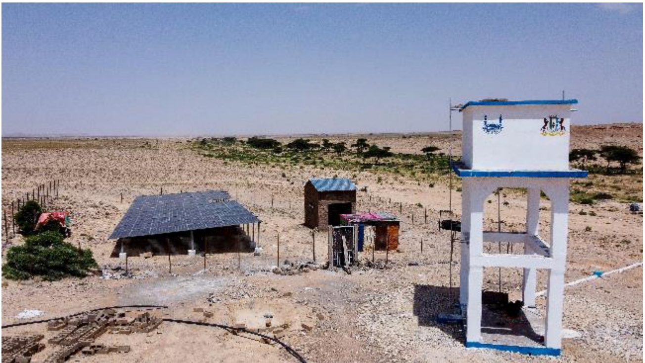
Figure 1: Solar Powered Borehole Pumps in Somalia
