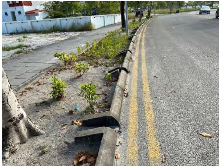
Implementation of infiltration drainage facilities without using a piped drainage system in Hulhumale (Source: MoE 2021)
