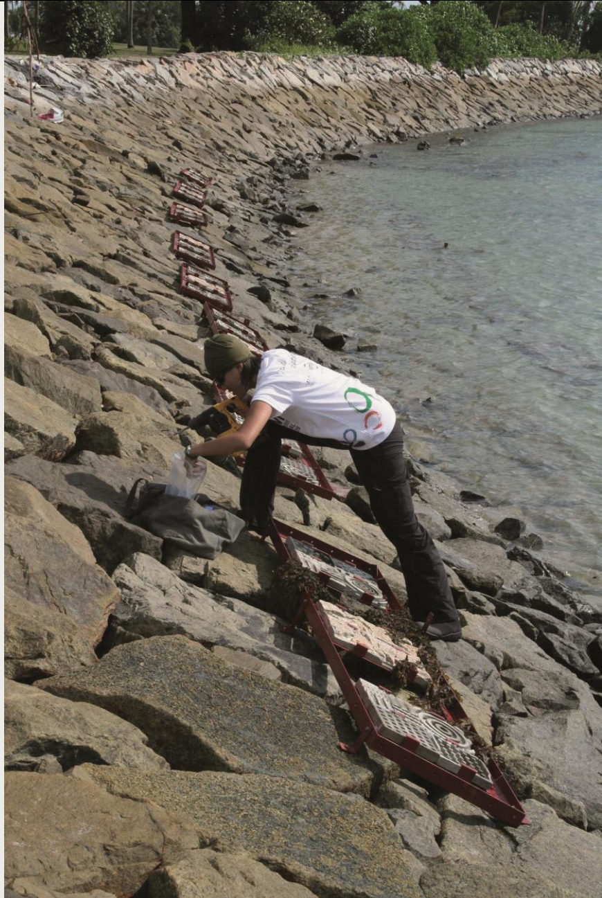
Multi functional coastal revetment placing habitat-promoting tiles in Singapore similar settings can be used eg: breakwater, seawall or groynes for example specifically painted tiles to attract corals and other sessile organism in a breakwater
